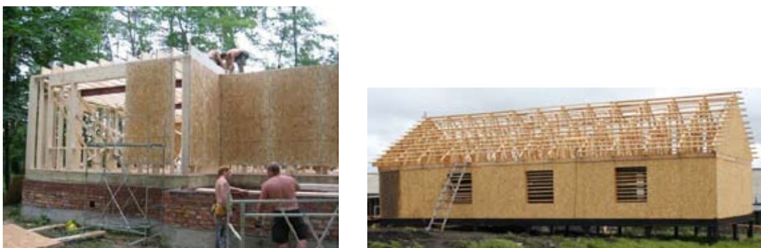
Fig. 11. Erection of the house in Nosok with the help of frame panel technology
