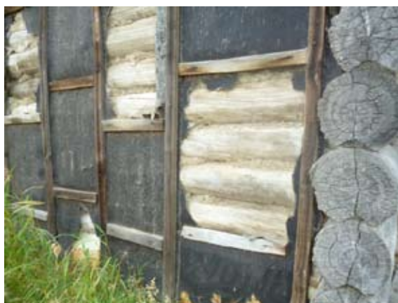
Fig. 10. The photograph of the damage of wall covering
