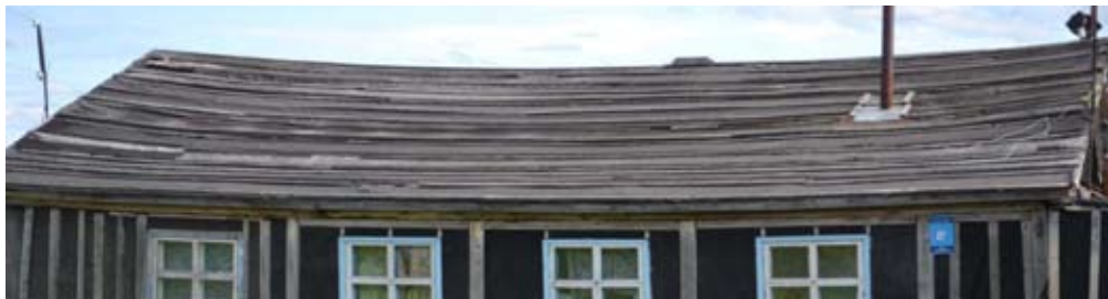
Fig.9. A photo of curvature, loss of the roof structure stability and damage to the roof coat
