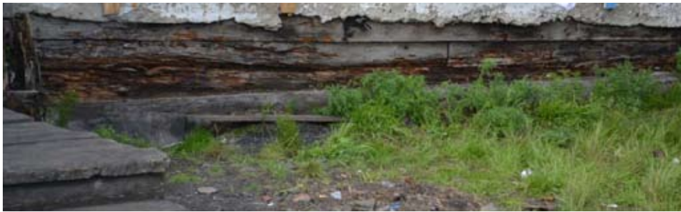
Fig. 8. A photo of beam structural decay under the influence of atmospheric precipitation
