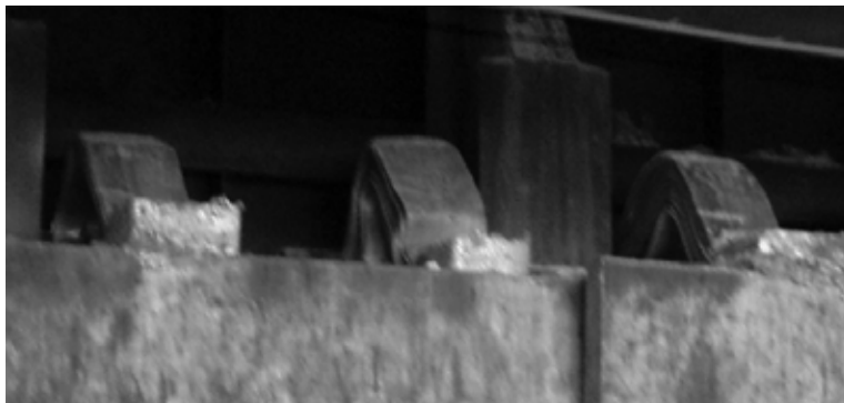
Fig. 5. Typical flexibles to busbar welds
