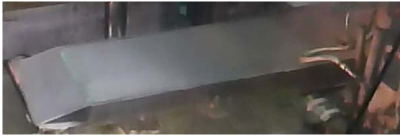
Fig. 6. Excessive cladding plate deformation
