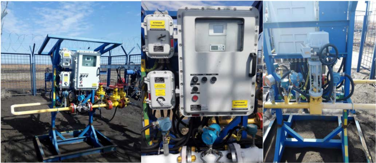
Figure 2—Gaslift automated process control system
