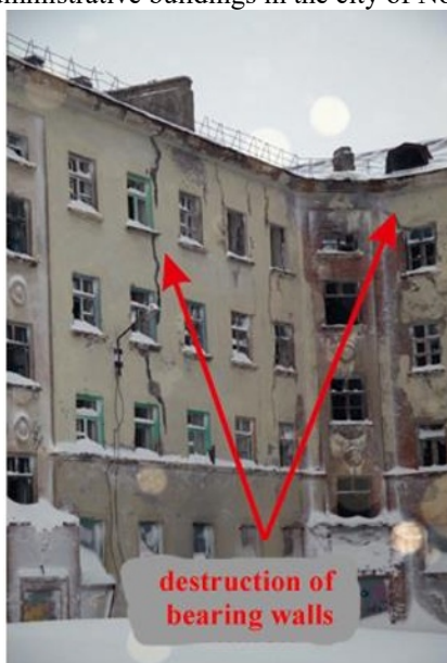
Fig. 7. Destruction of residential buildings in the city of Norilsk
